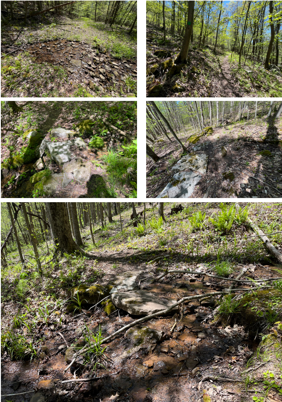
Typical tread conditions and acute drainage issues in the North Zone
